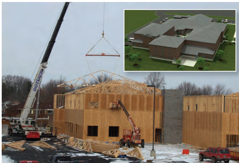
The Hendricks County Community Foundation continues to support Sheltering Wings which provides emergency housing for all women and children suffering from any form of domestic abuse. Pictured above is the expansion project in March 2011 and a conceptual drawing of the expansion. In 2010, HCCF awarded Sheltering Wings a $10,000 grant from the Deedee Daniel Opportunity Fund for their new expansion and a $25,000 grant from the Anderson Family Fund for general operating expenses.
